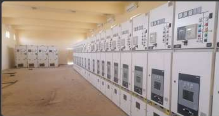
Umm Qasr Electrification
